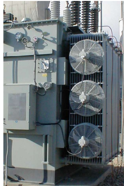
Figure 29 – Cooling Fans on a Niagara transformer
